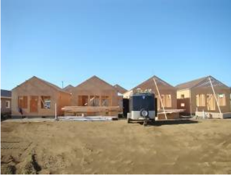
Front view of the Shops that front Pt Brown Ave. (Units #A - #D, left to right).
