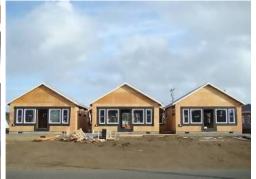
View of the Shops that front Minard Ave w/ a concrete sidewalk poured in front of the shops.
