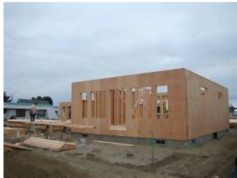
Front view of Unit #G.
