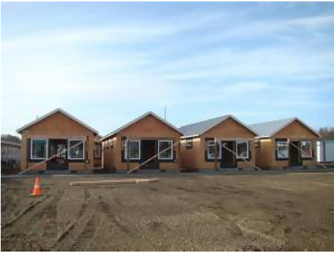
View of the Shops that front Pt Brown Ave w/ a concrete sidewalk poured in front of the shops.
